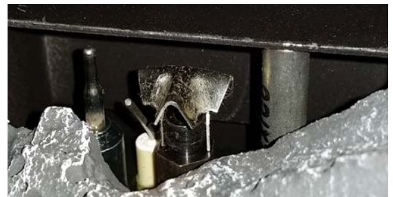
Figure 21: Pilot assembly beside the burner.
