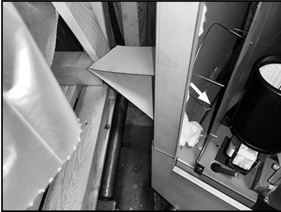
Figure 32: Rating label in place.
